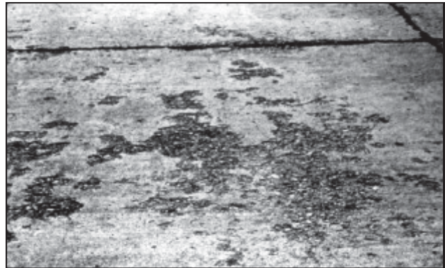
Scaling on Concrete Slab
